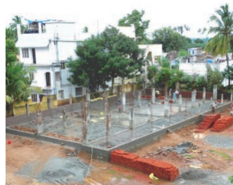
Michaelas (top photo with hands in pockets) is managing the construction of the new boys' dormitory and study hall. It should be ready for Easter. All donations welcome!
